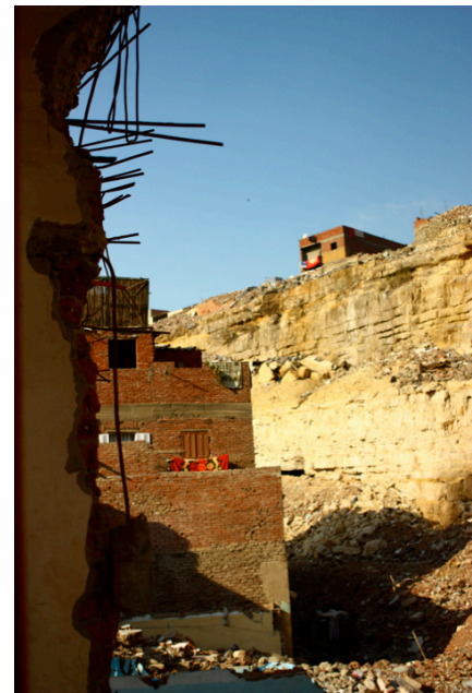
Figure 3. Foreground shows the wall of an inhabited home cut in half during a government demolition (credit: M. Hutchison)
